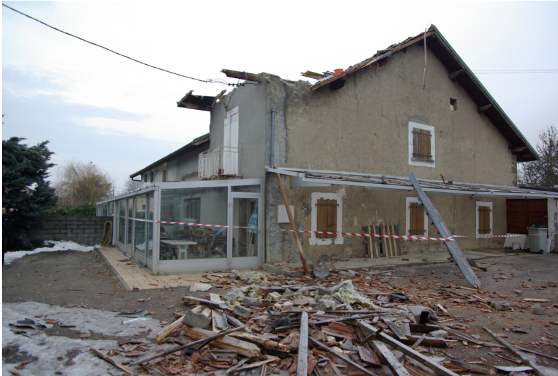
Figure 2 - Damage to the house
