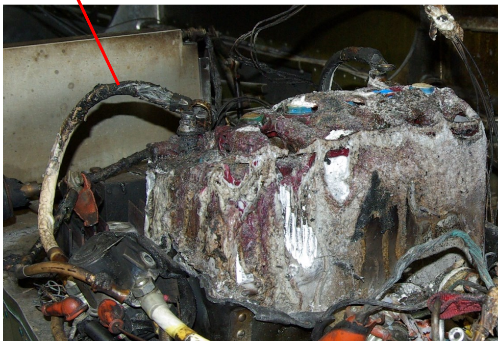
Figure 65: Conductor associated with positive terminal of battery Source: BEA
