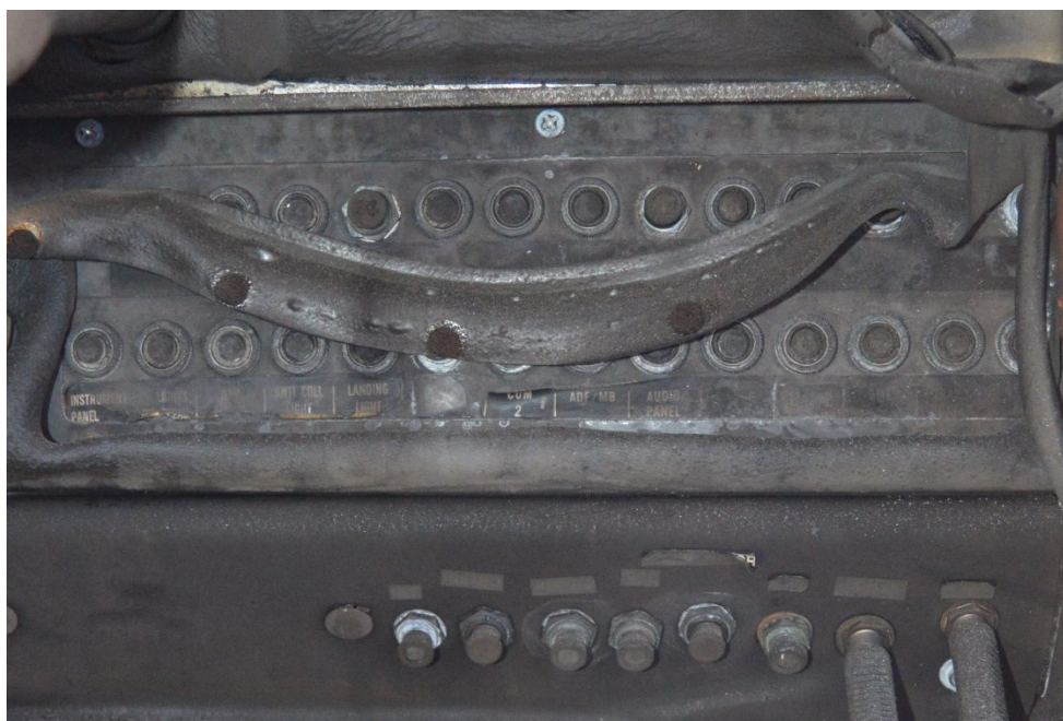
Figure 6: Circuit breakers on instrument panel Source: BEA
