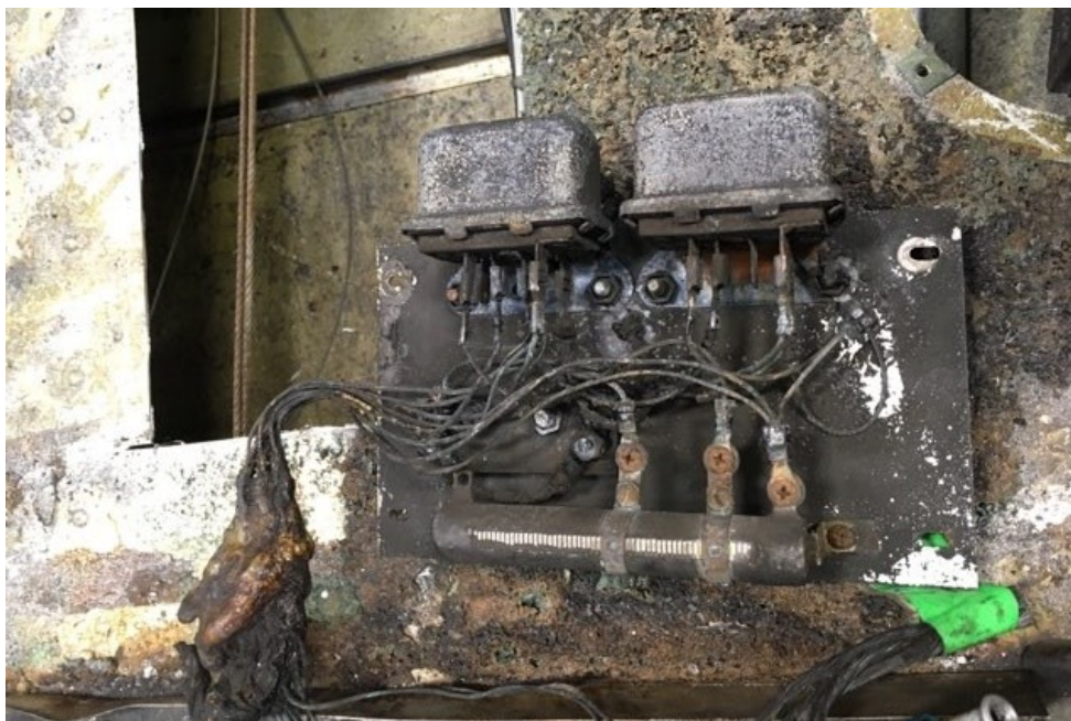
Figure 32: Electrical assembly removed from right partition Source: BEA
