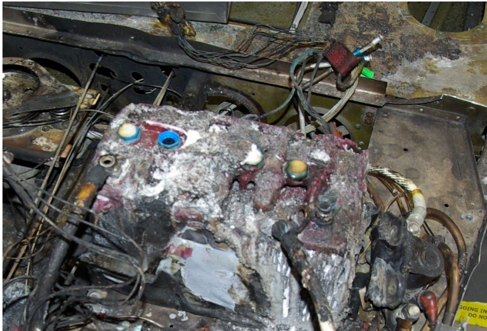
Figure 48: Battery Source: BEA
