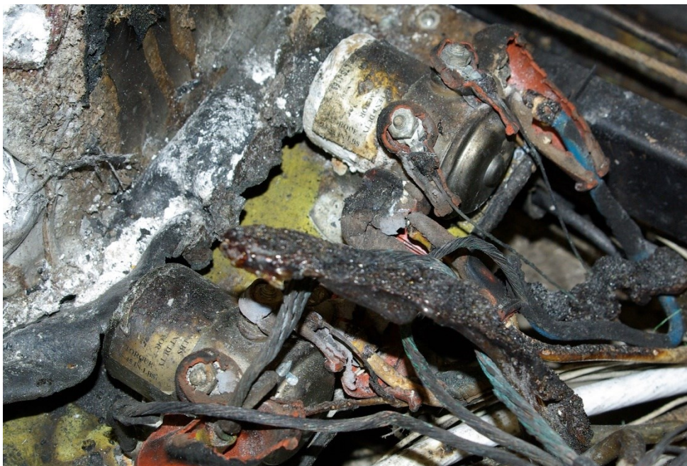
Figure 31: Contactors situated in front of battery Source: BEA
