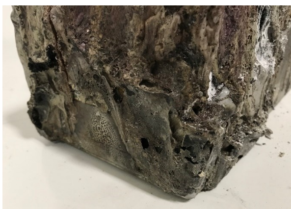
Figure 50: Lower part of battery, positive terminal side Source: BEA
