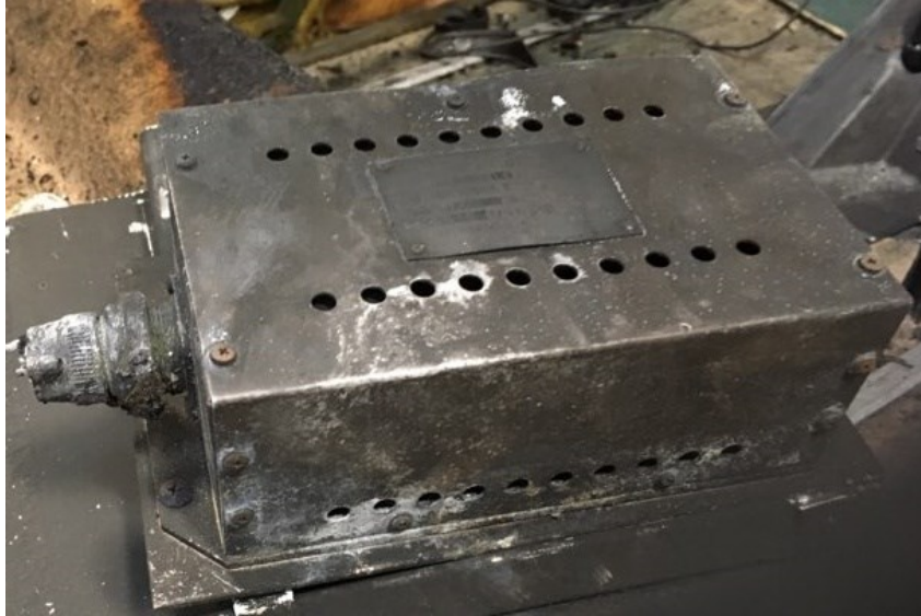
Figure 33: 12 V - 24 V converter removed from right partition Source: BEA
