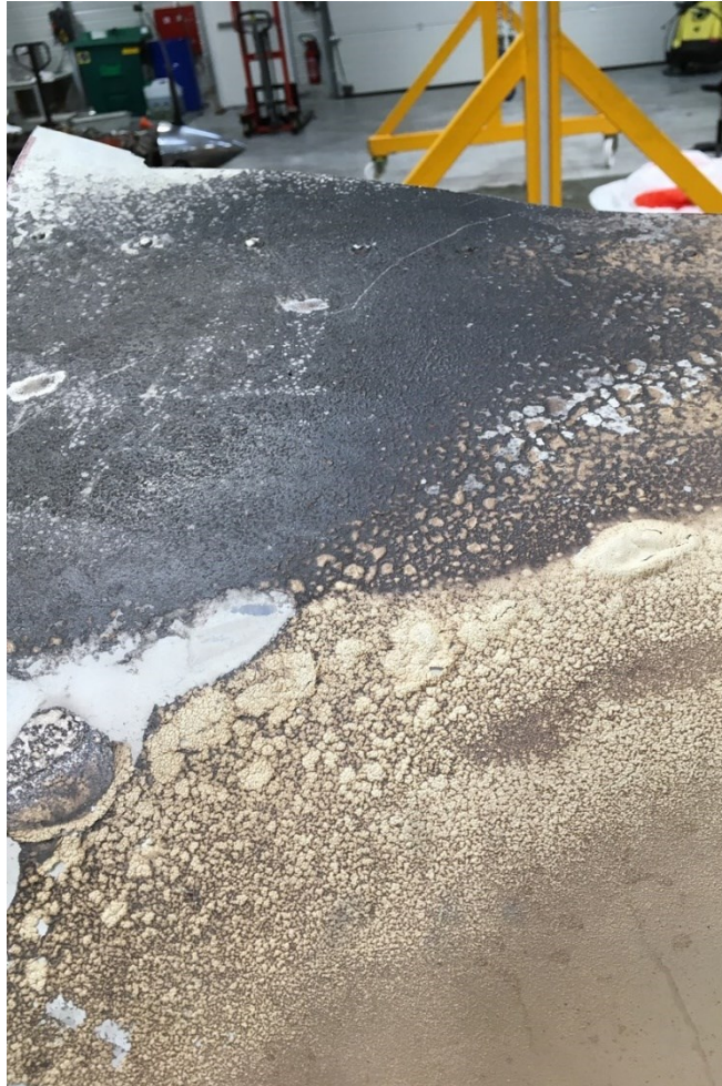
Figure 12: Detail of condition of external paint Source: BEA
