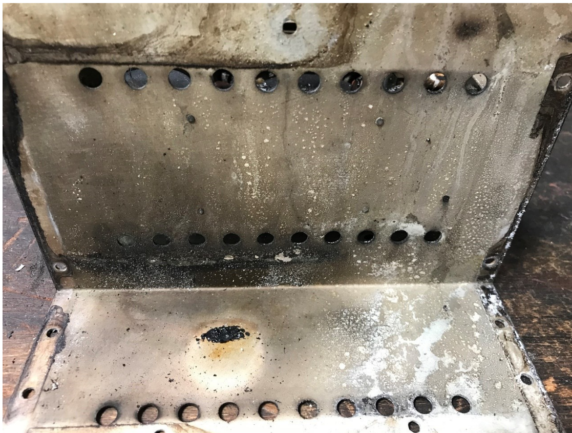
Figure 35: Inner surface of 12 V - 24 V converter casing
