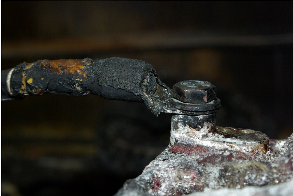
Figure 52: Negative terminal of battery
