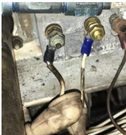
Conductors connected to the ammeter, located behind the instrument panel
