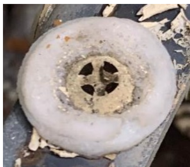
Softening of insulating washer
