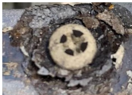
Destruction of insulating washer
