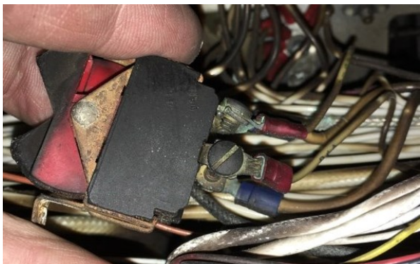
Conductors connected to master switch, located behind instrument panel
