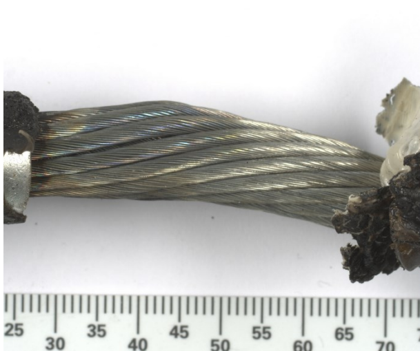
Figure 67: Bluish colouring of conductor (overheating of conductor) Source: BEA
