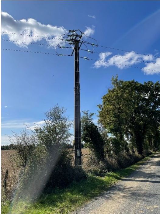
Figure 2: one of the two poles either side of the accident site (source: BEA)
