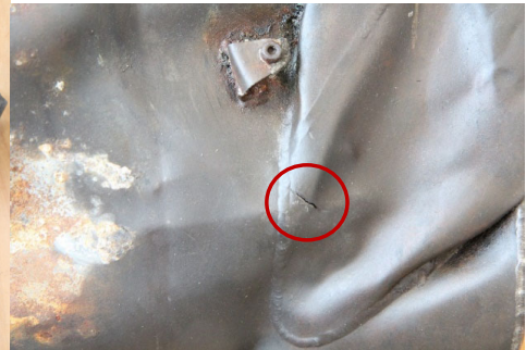
Figure 3: View of the crack
