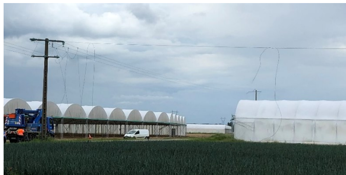
Figure 4: branch-off pole and severed cables (Source: BEA)
