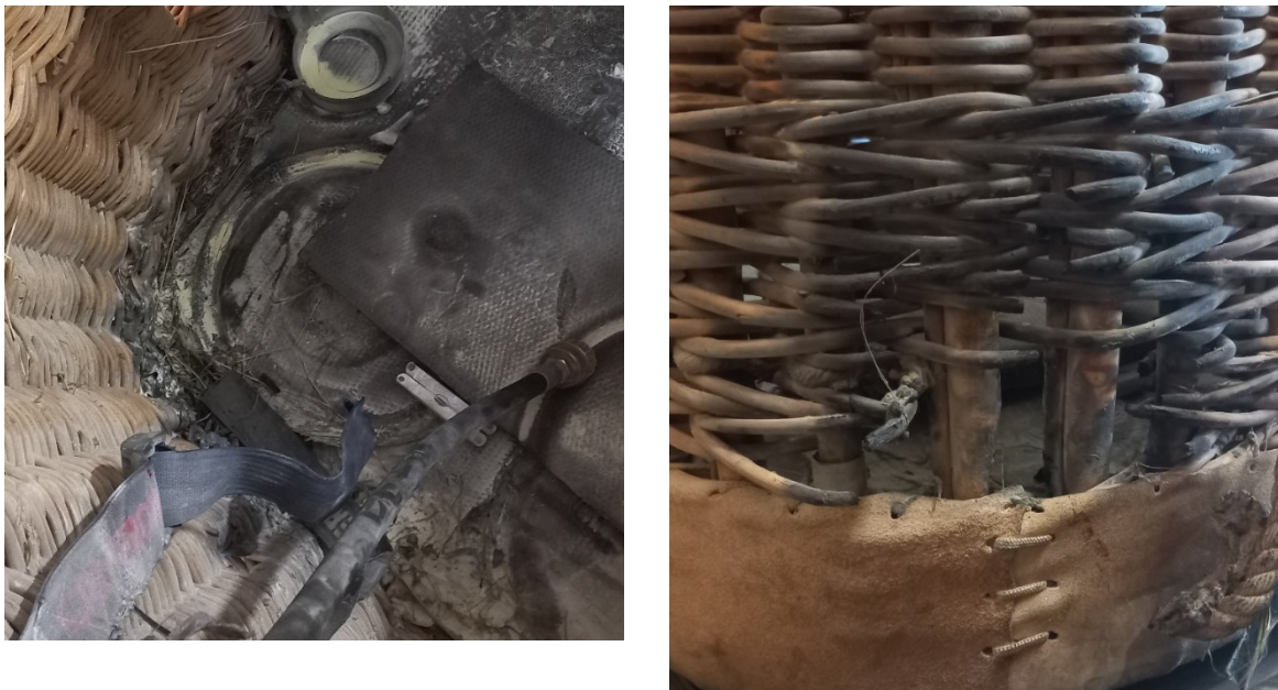
Figure 2: views from interior and exterior of burnt areas of pilot's compartment (Source: BGTA)
