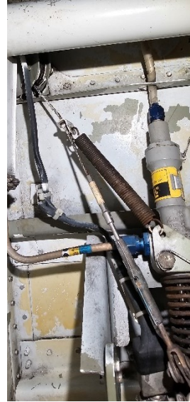
Figure 6: no anti-corrosion protection (yellowish in colour) on the walls of the nose landing gear well (Source: R&O)
