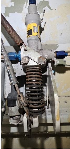
Figure 5: signs of corrosion on springs of nose landing gear mechanism 22 (Source: R&O)
