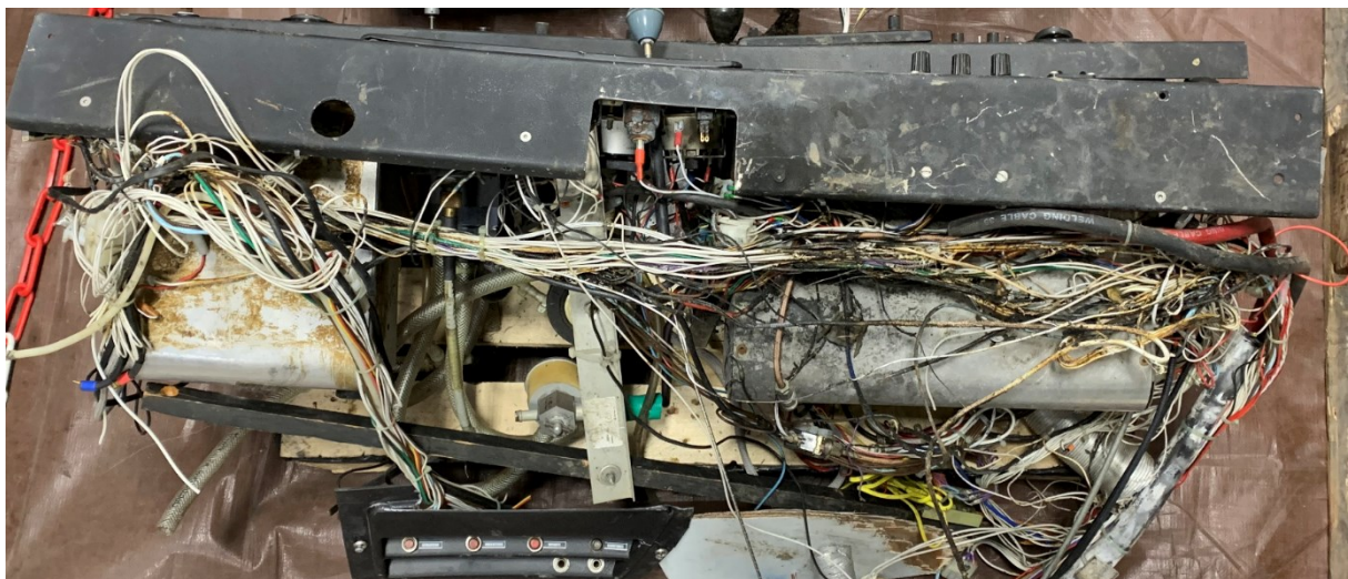
Figure 1: back of the instrument panel and location of overheating marks (Source: BEA)
