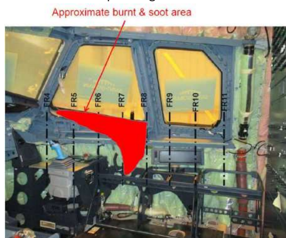
Figure 17: corresponding area on an A320 (source: BEA/EEAID)
